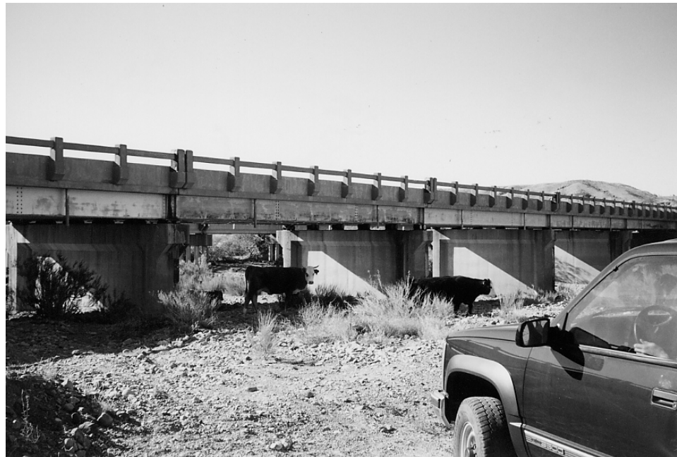
Figure 4-23: Side view of the third northern span of the Alamosa Canyon Bridge
